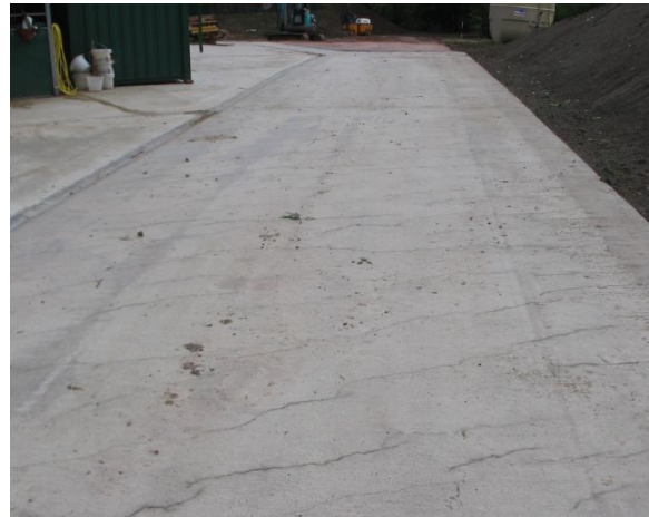
Plastic shrinkage cracking
